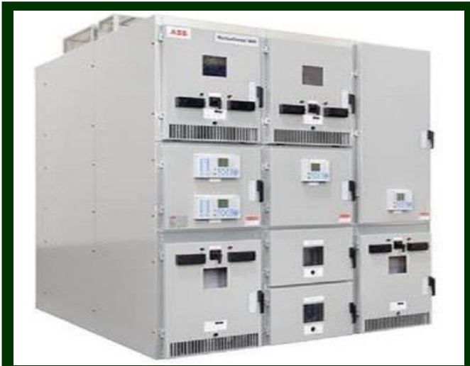
MEDIUM VOLTAGE SWITCHGEAR
